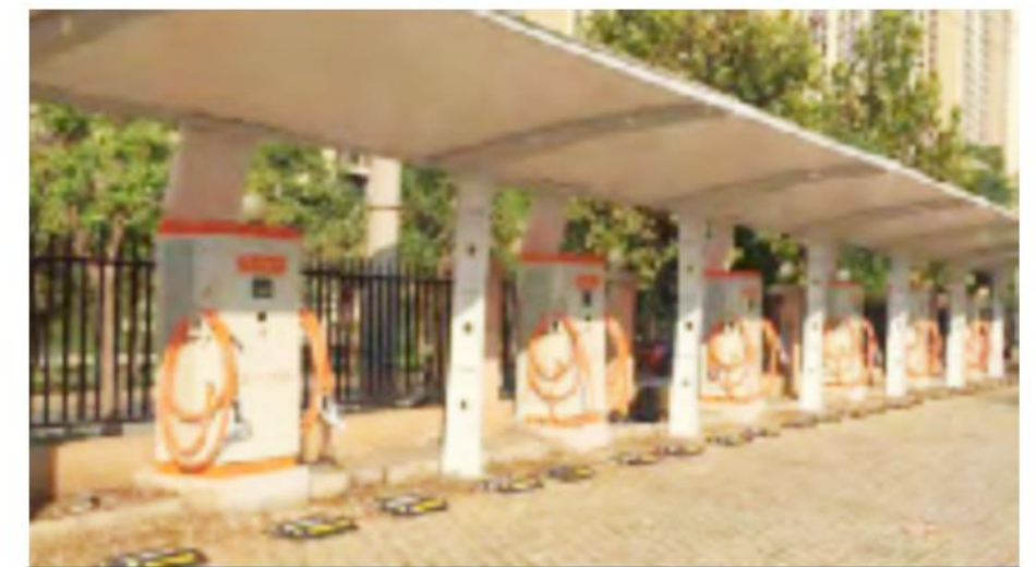
XiaoJu Public Charging Station
