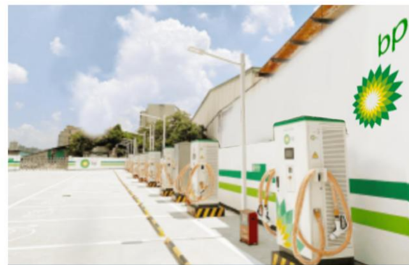
BP Public Charging Station
